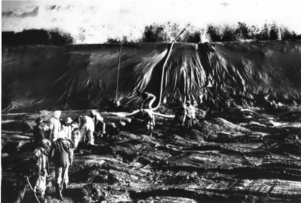
57 Beach mining for diamonds in South West Africa. Movable interlocking concrete blocks, with specially designed cavities to dissipate the force of the waves, stand behind the plastic-covered sand supporting wall.
